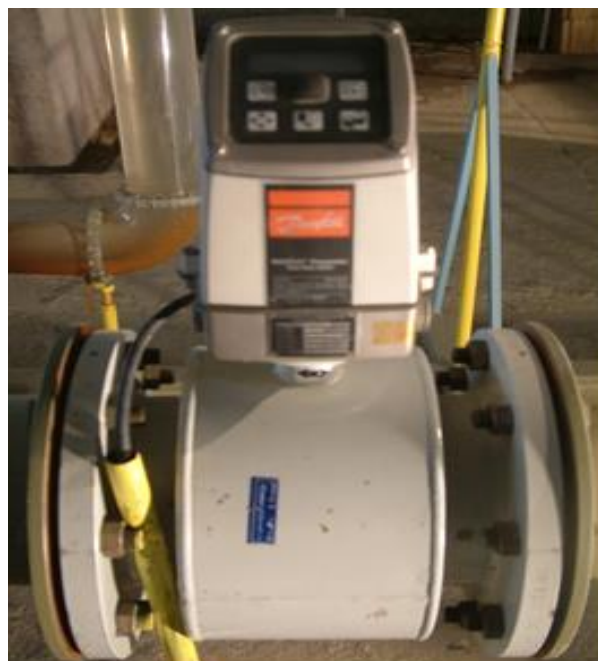
Fig. 5. Flowmeter installed in the model
